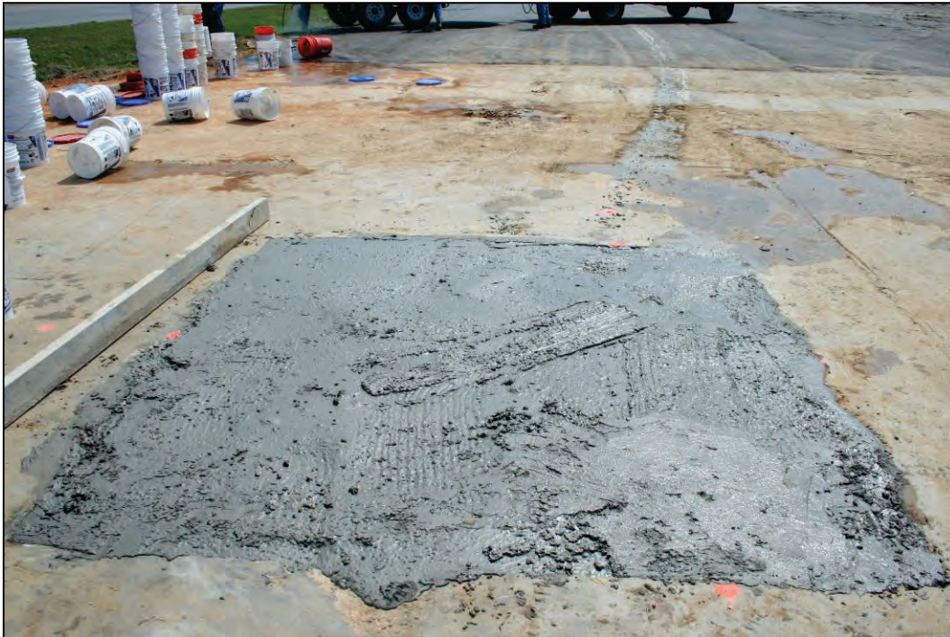
Figure 1. Inadequate concrete pavement repair surface.
